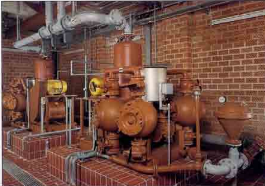
Spherical Membrane Pumps in a municipal wastewater treatment plant
